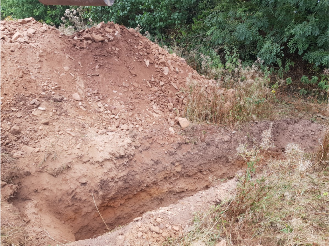
Number: TP15 Project Glounthaune Housing Phase 2 Project No P18170 Engineer AECOM
