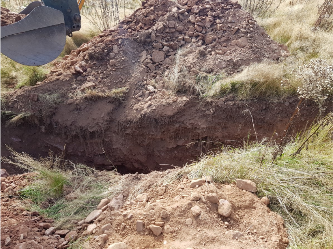
Number: TP03 Project Glounthaune Housing Phase 2 Project No P18170 Engineer AECOM
